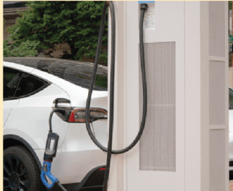
EV Charging Point
