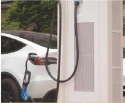
EV Charging Point
