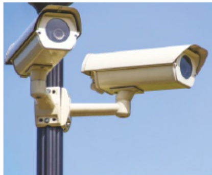
4X6 CCTV Surveillance
